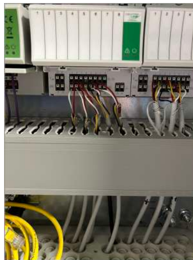
Figure 6A. A part of cable connection between temperature sensors and CentraLine NX software
